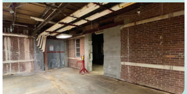
The original hospital exterior wall and window exposed during the demolition phase of the Surgical Pavilion renovation project.
